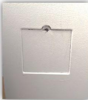
Heater access panel
